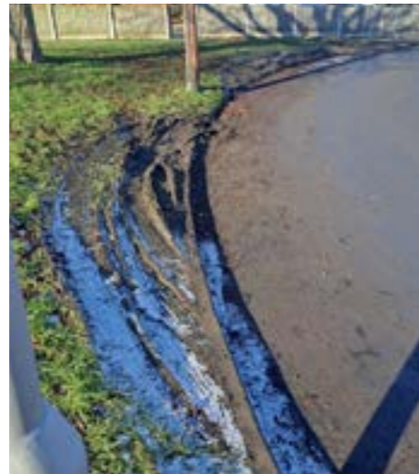
Greystones Drive, Ossett - trip to rail prevent damage to grass verges and access issues by vehicle parking.
